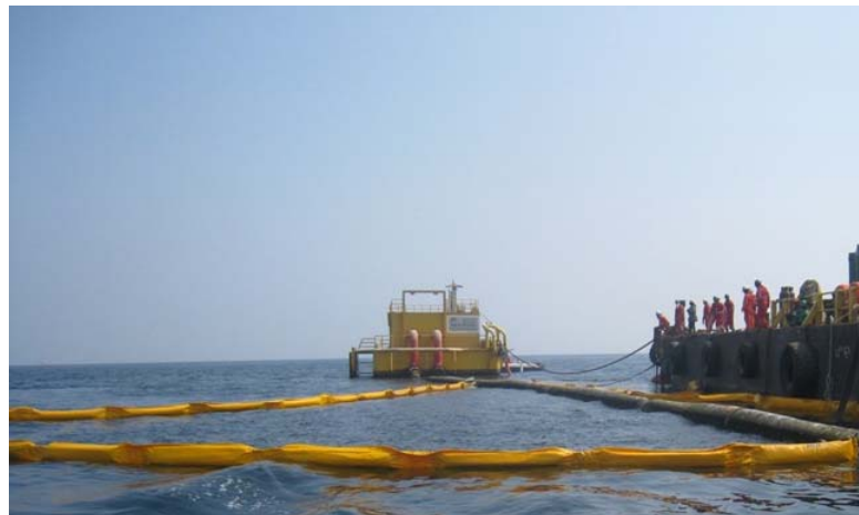
SESME supporting VHFL with offshore oil spill response services during routine maintenance operations
